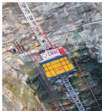
PMH at Pump House, Kaleshwaram
