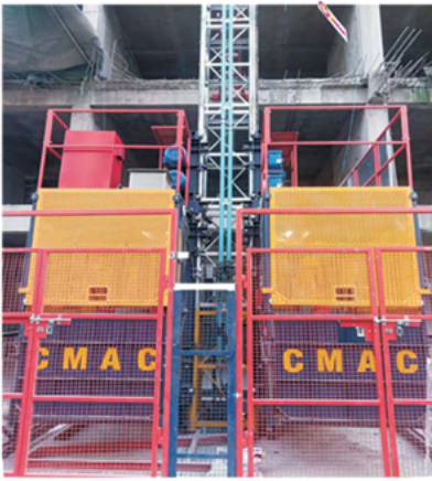
PM Hoist Double Cage, Hyderabad
