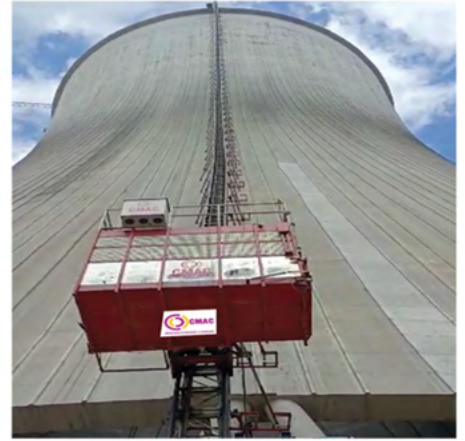
Curved Hoist Bangladesh
