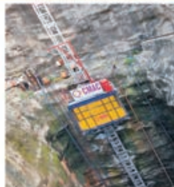
PMH at Pump House, Kaleshwaram
