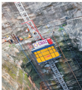
PMH at Pump House, Kaleshwaram
