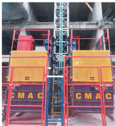
PM Hoist Double Cage, Hyderabad
