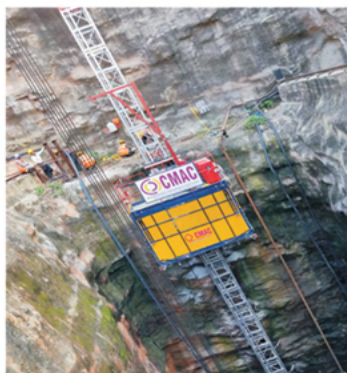
PMH at Pump House, Kaleshwaram
