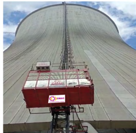
Curved Hoist Bangladesh
