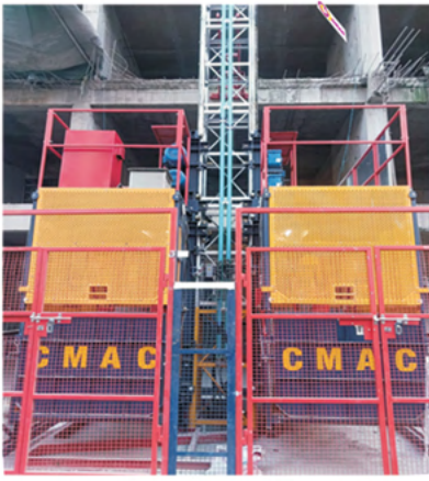
PM Hoist Double Cage, Hyderabad
