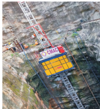
PMH at Pump House, Kaleshwaram
