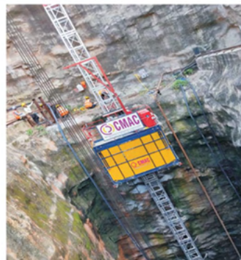
PMH at Pump House, Kaleshwaram
