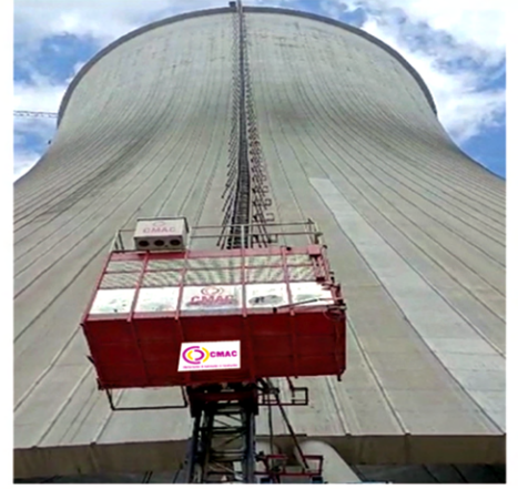
Curved Hoist Bangladesh
