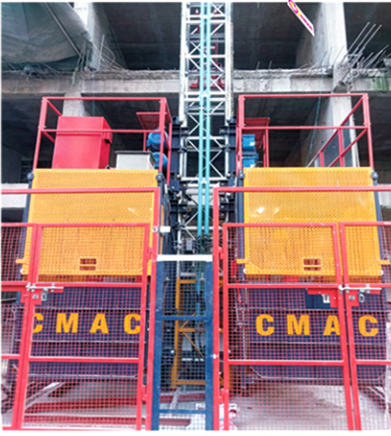
PM Hoist Double Cage, Hyderabad
