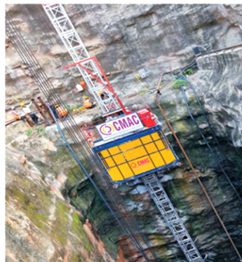
PMH at Pump House, Kaleshwaram
